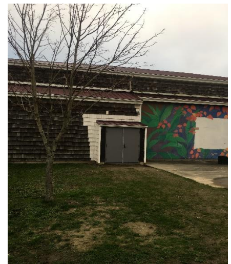
ES COURTYARD NEW RISER ROOM
